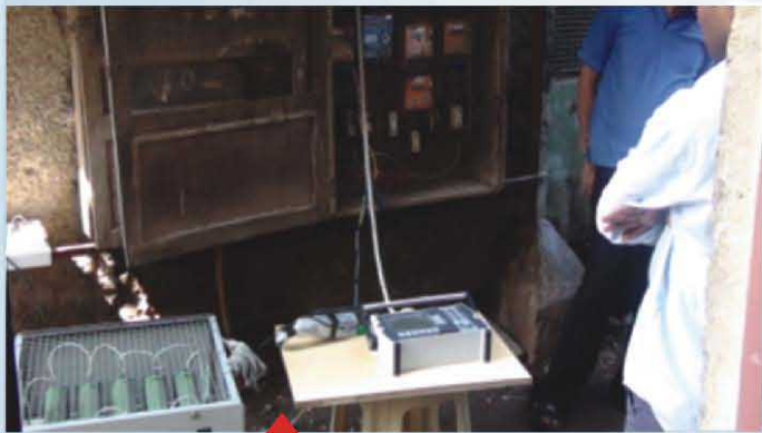
Calibration of Energy Meters for Reliance Consumers as requested by Maharashtra Electricity Regulatory Commission.
